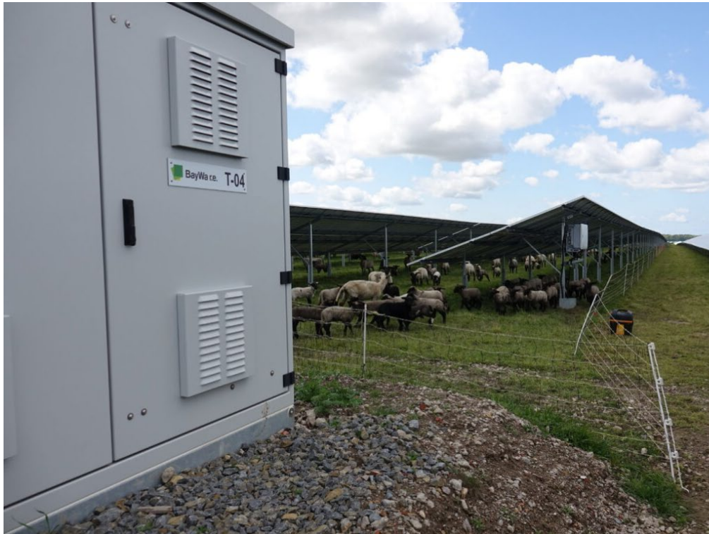
Plate 3: Typical transformer on a solar farm site
